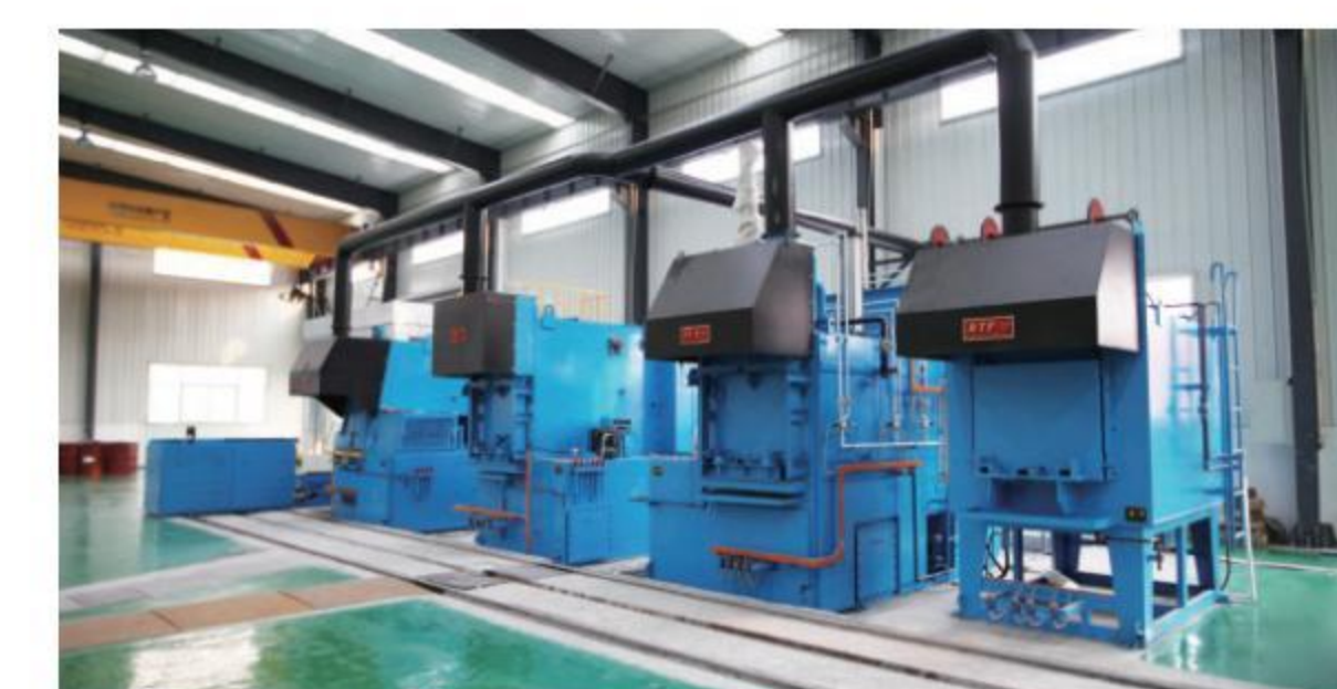
渗碳炉 Production equipment
