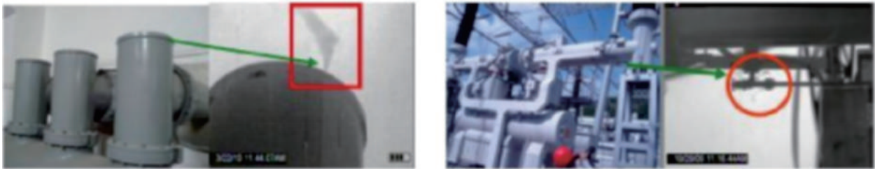
Gas leaking detection
